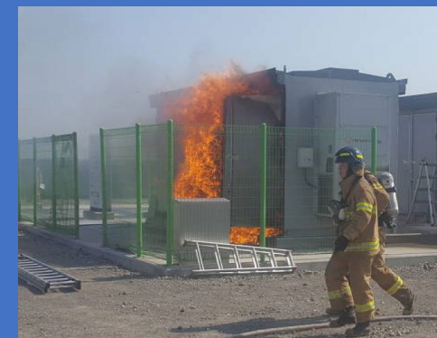
ESS (Energy Storage System)
