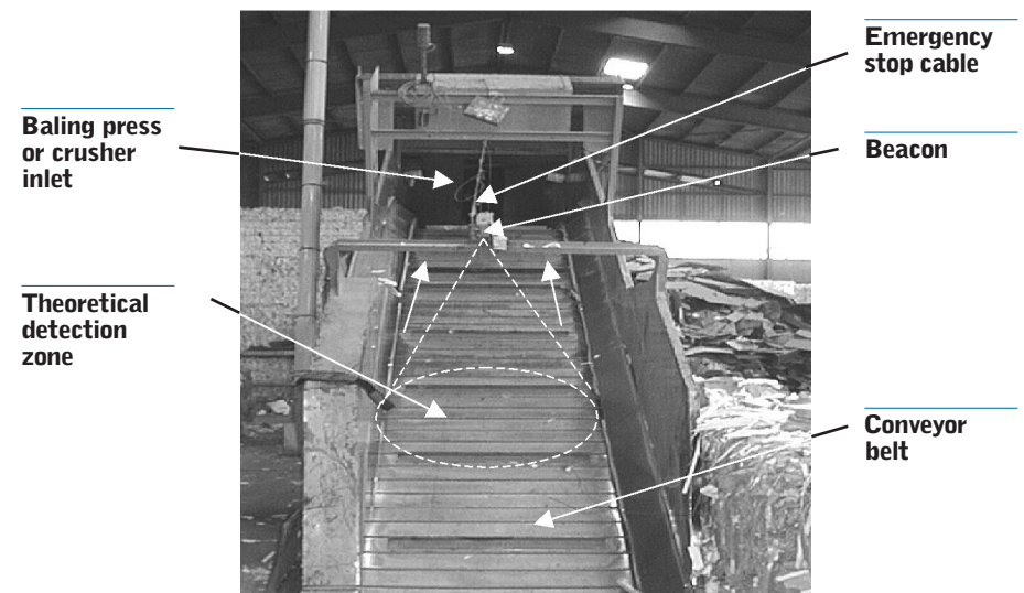
Fig. 5. Typical implementation of radio wave detection system on conveyor.
